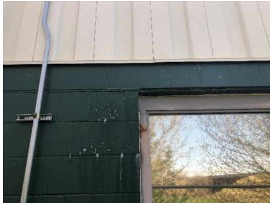
West elevation efflorescence
