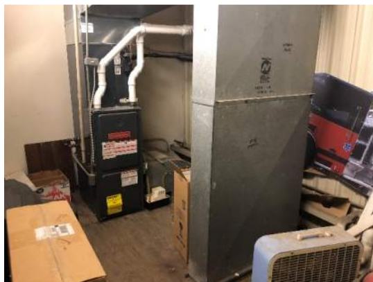
Furnace room on mezzanine
