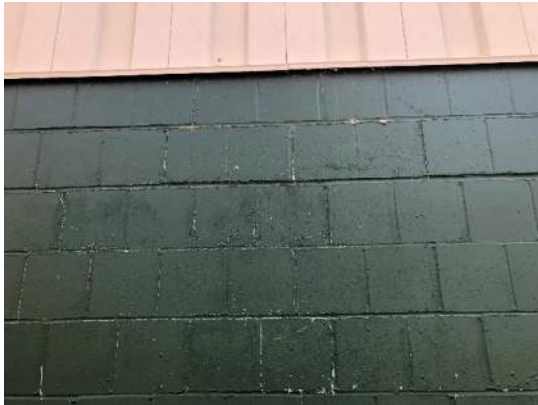
West elevation efflorescence
