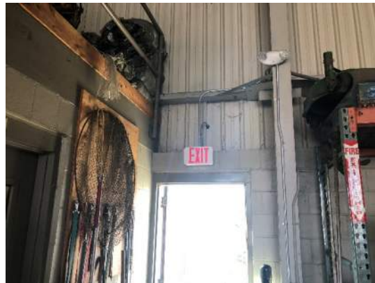
South wall efflorescence
