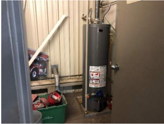
Furnace room on mezzanine
