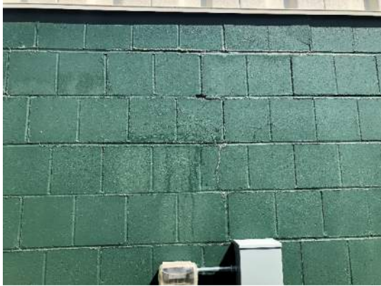
South elevation missing mortar
