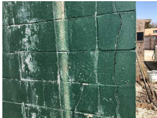
Cracks in all corners
