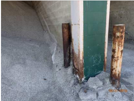
29. View of damage at base
