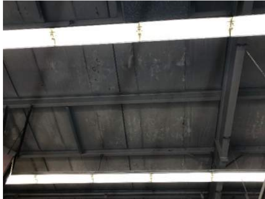
West bays water damage
