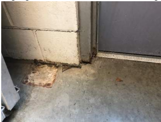
Rusted frame in dog cage room
