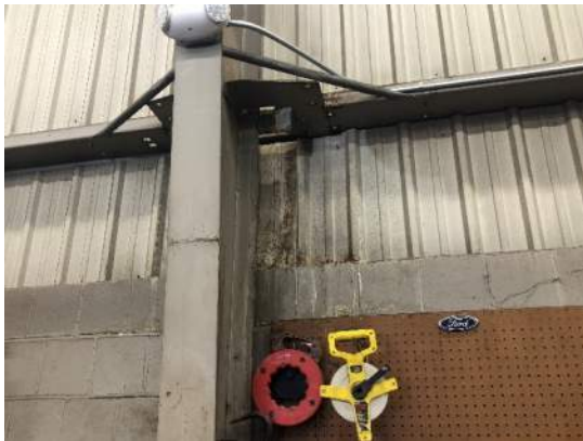
South wall efflorescence and water damage
