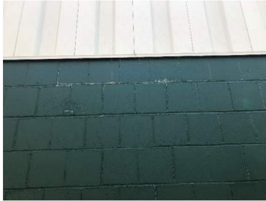
West elevation efflorescence
