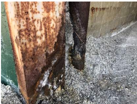
Rusted opening steel
