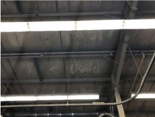
West bays water damage
