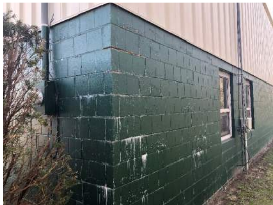
NW corner efflorescence and missing mortar
