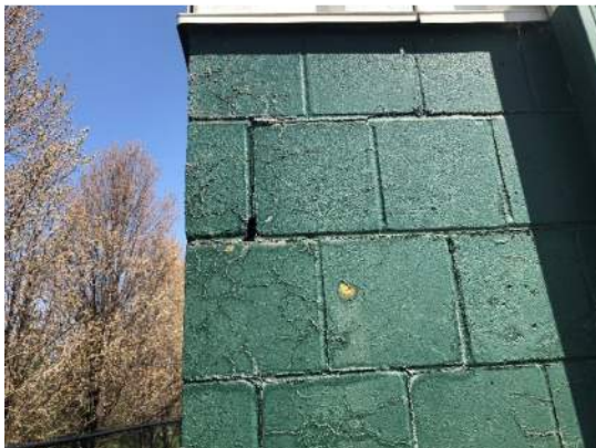
SW corner missing mortar
