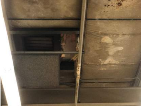
West bays water damage
