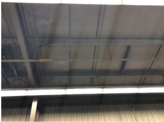
East bay's water damage
