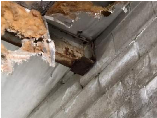
Salt building distressed steel supports
