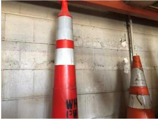
South wall efflorescence
