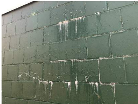
West elevation efflorescence
