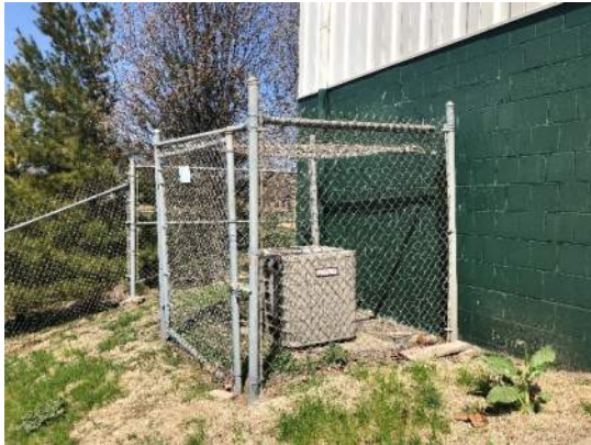
SW corner condenser
