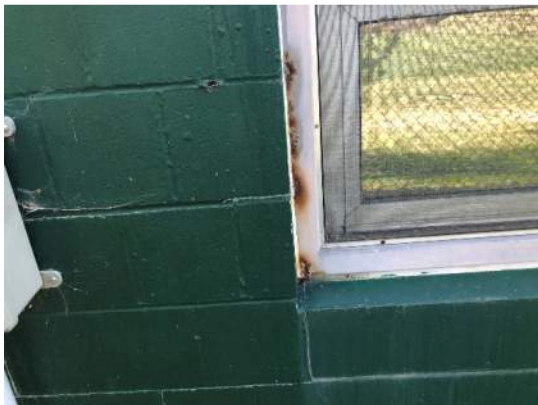
West elevation rusted frame
