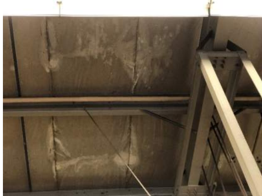
West bays water damage
