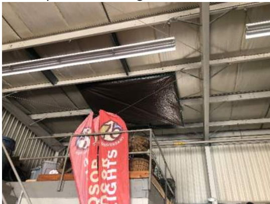
East bays water damage
