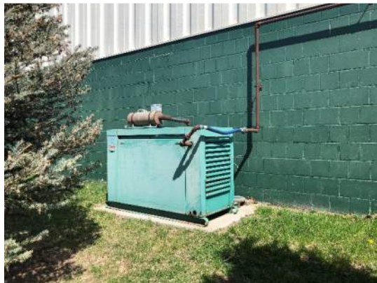
South elevation generator
