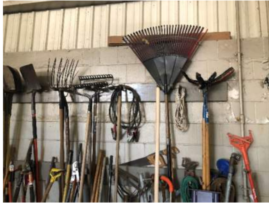
South wall efflorescence
