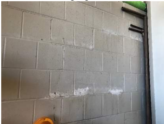
East wall efflorescence
