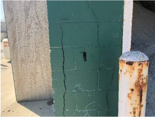
Cracks in all corners
