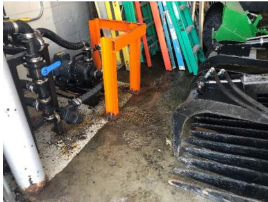
NE corner at brine pump
