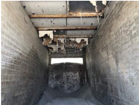
Salt building distressed materials
