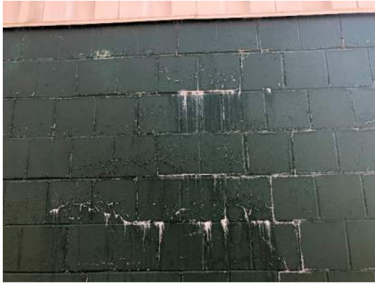
West elevation efflorescence
