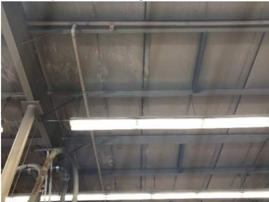
East bay's water damage
