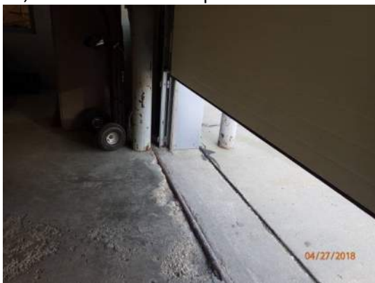
19, 20. View of concrete in need of repair
