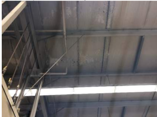
East bay's water damage
