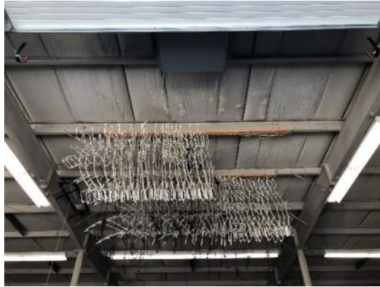
East bays water damage
