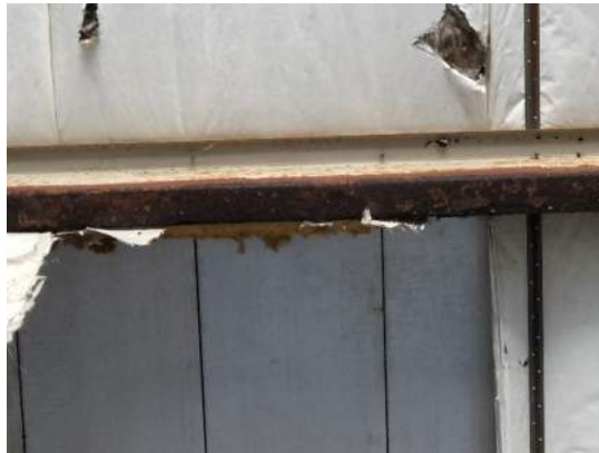
Salt building distressed roof structure
