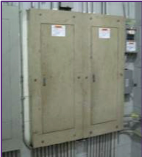
MANY ORIGINAL ELECTRICAL PANELS STILL EXIST
