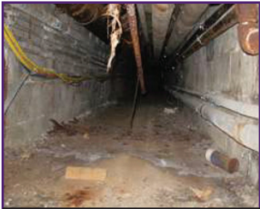
UTILITY DISTRIBUTION TUNNEL HAS BEEN FLOODED NUMEROUS TIMES
